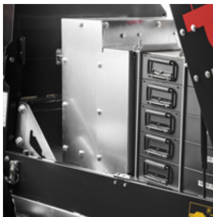
21 kWh De lithiumbatterij (Li-ion, 65VDC, NMC)
