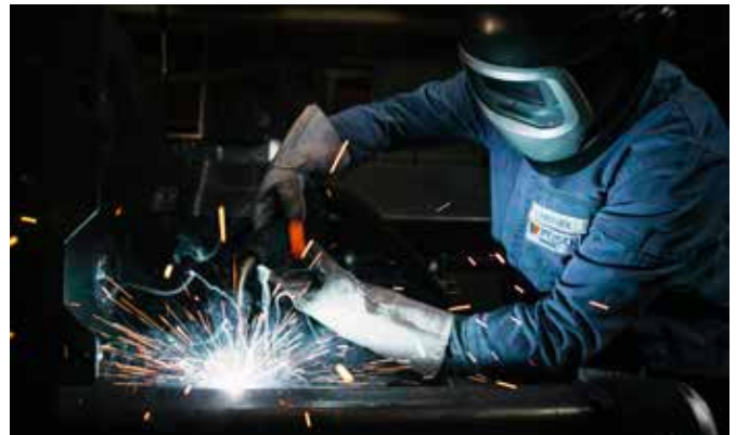
Our experienced welders, qualified according to DIN, ensure the highest quality of the welded structures every day.
